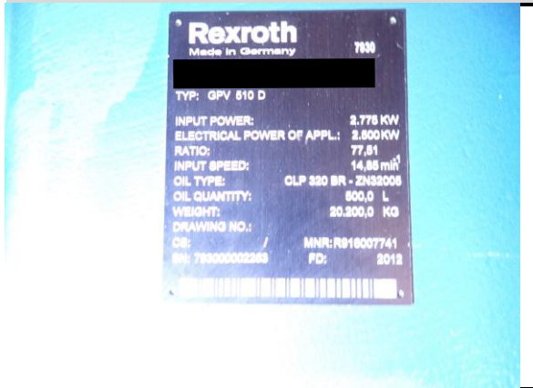
Photo of gearbox nameplate
