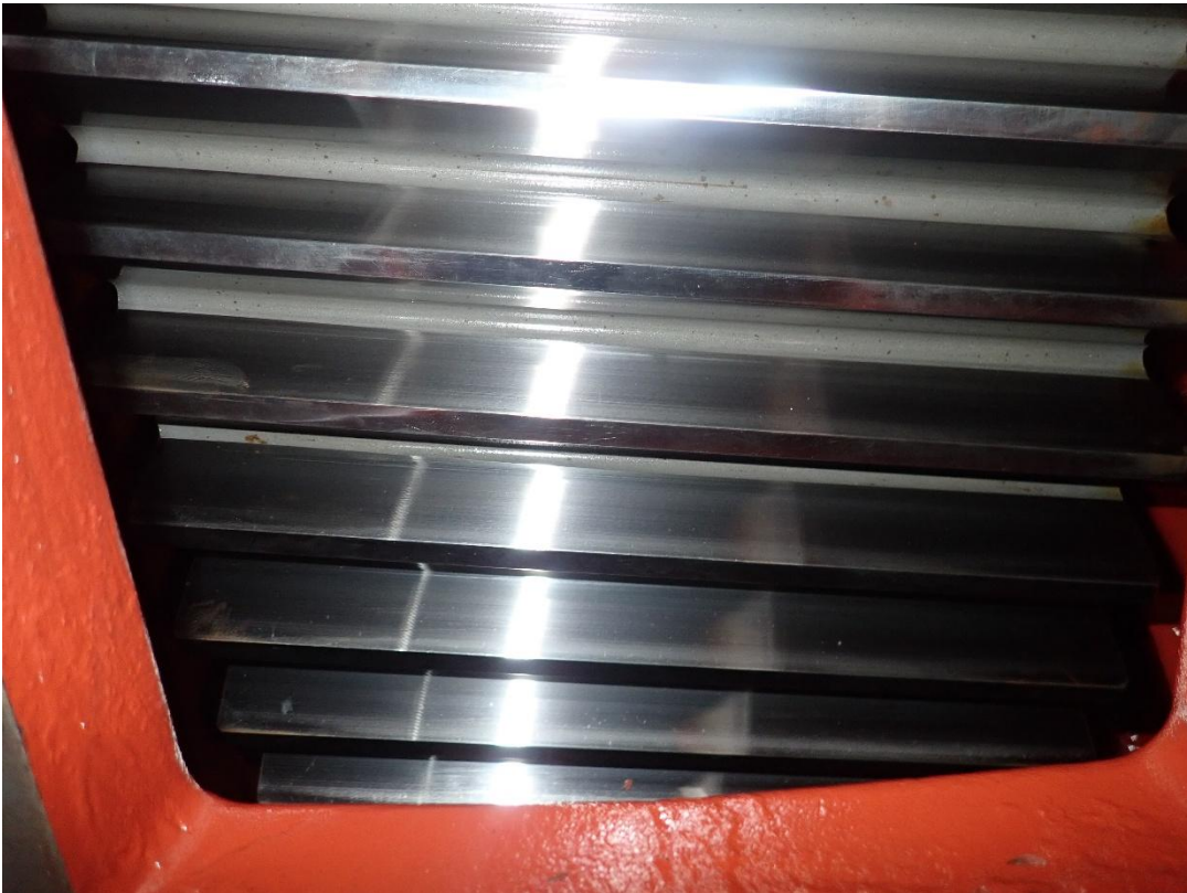
Photo 2: Output shaft, gear. No deviations have been observed.
