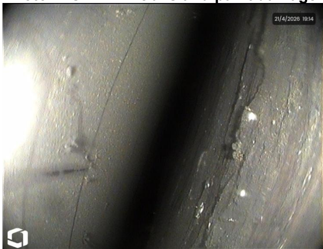
Photo 3: Coil 24 Debris and burn surface.
