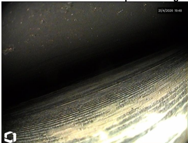
Photo 11: Coil 32. Debris and paint damage.
