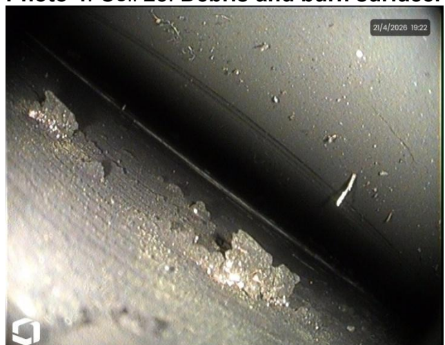
Photo 6: Coil 27. Debris and burn surface.
