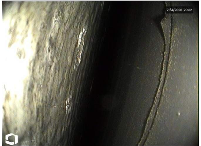
Photo 16: Coil 37. Debris and paint damage.
