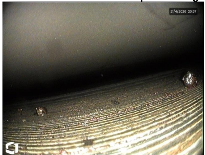
Photo 24: Coil 45. Debris and paint damage.
