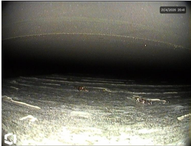
Photo 19: Coil 40. Debris and paint damage.
