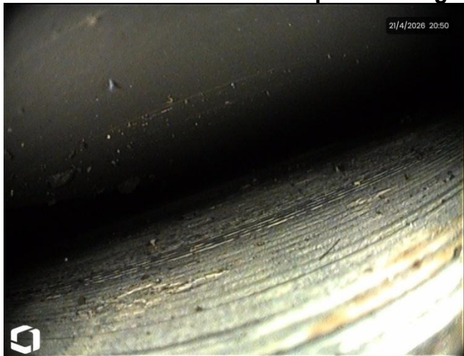
Photo 21: Coil 42. Debris and paint damage.
