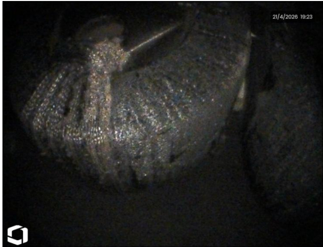
Photo 7: Coil 28. Debris and paint damage.
