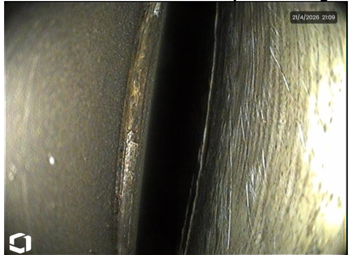
Photo 28: Coil 49. Debris and delamination.
