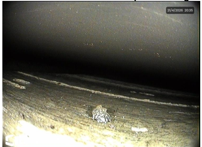
Photo 18: Coil 39. Debris and paint damage
