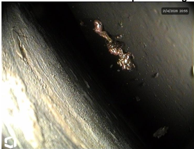
Photo 23: Coil 44. Debris and paint damage.
