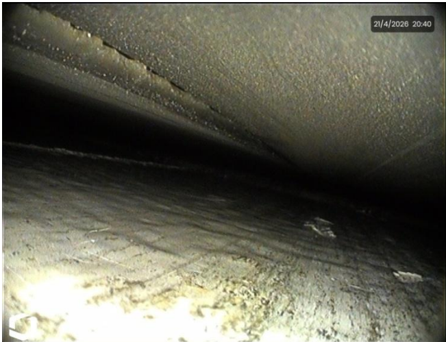
Photo 17: Coil 38. Debris and delamination.
