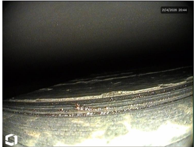
Photo 20: Coil 41. Debris and paint damage.
