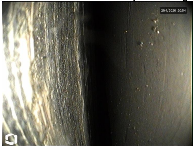
Photo 22: Coil 43. Debris and paint damage.
