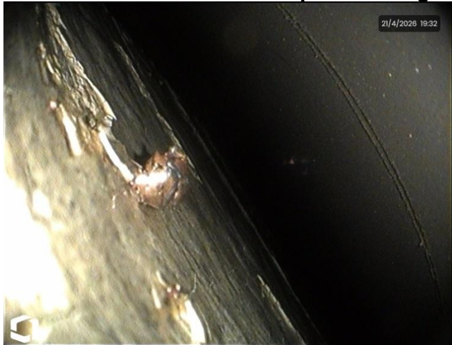
Photo 9: Coil 30. Debris and paint damage.
