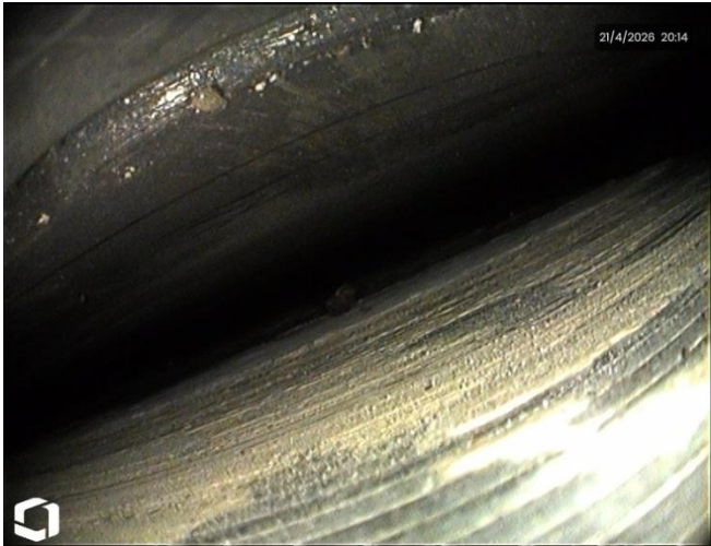
Photo 13: Coil 34. Debris and delamination.
