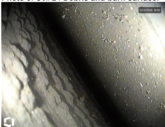
Photo 5: Coil 26. Debris and burn surface.
